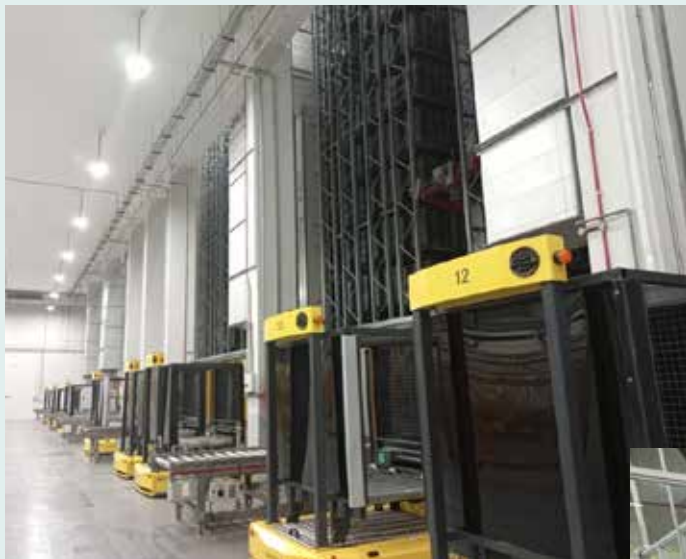
Movement of pallets of banknotes into and from the rack inside the vault managed by automated cranes.
